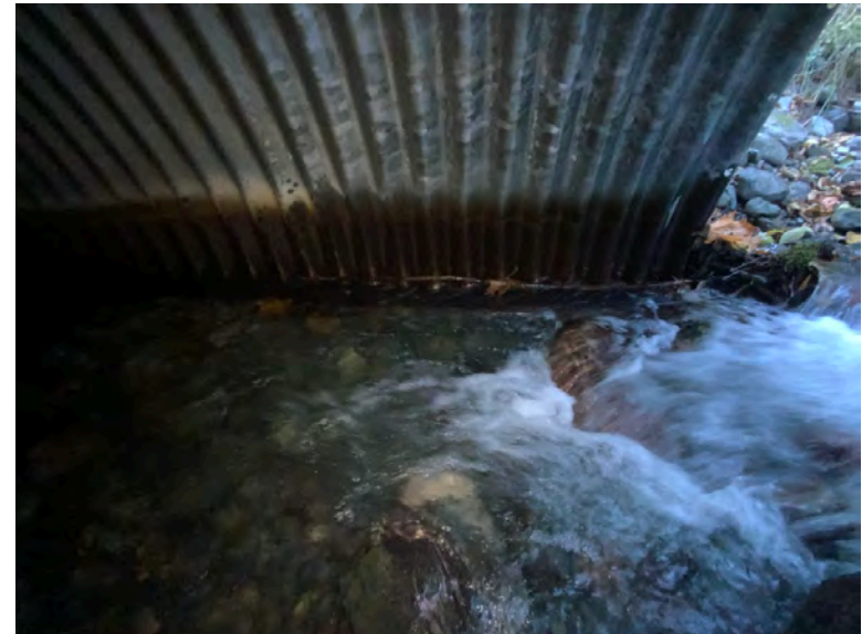
Right upstream footing erosion under footing.
